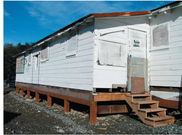
A view of the wing of the boathouse nearest the bridge, showing new foundation, October 2006.
